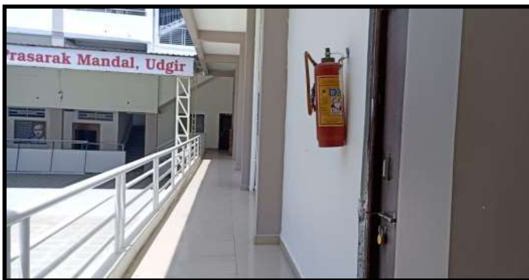
Fire Extinguisher Facility
