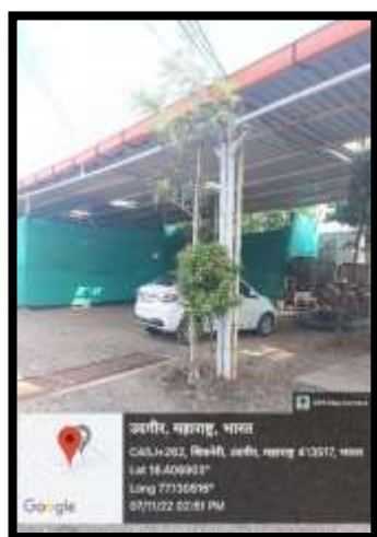
Rain Water Conduction PVC Pipes
